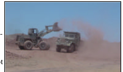
2.5 yd bucket loader filling a 5 ton dump at the burrow site. Picture by 2LT Shaunte Chandler
