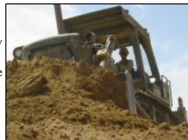
SPC William Stoltenberg stockpiles fill material at the borrow pit. Picture by 1LT Brian Meister.
