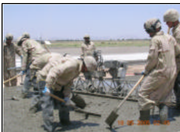
1st Platoon places concrete at the Mobility Ramp at KAF Picture by 1LT Jennifer Austin
