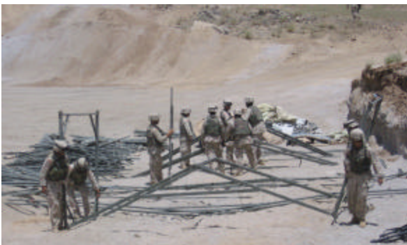
A squad of Kodiak Soldiers work on setting up the first of several 36 meter long tents; Photo by CPT Kim Gage
